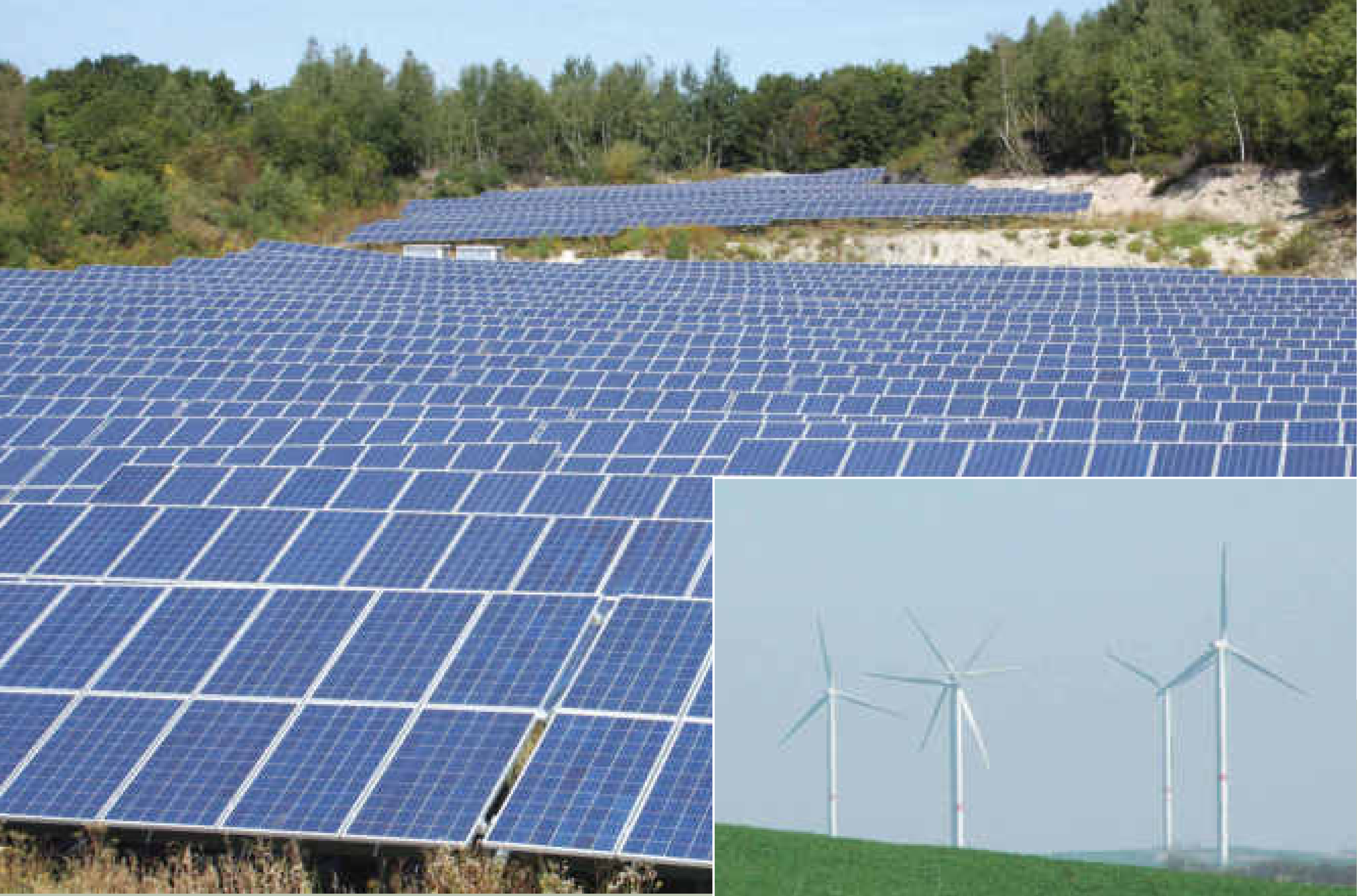
Photovoltaik-Anlage in Gersheim © Anita Naumann
